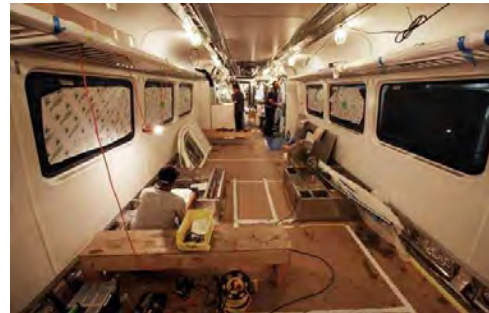
Technicians fit out the interior of a Silverliner V railcar under construction at the Hyundai Rotem plant on Weccacoe Avenue in South Philadelphia. Photo by Laurence Kesterson.
