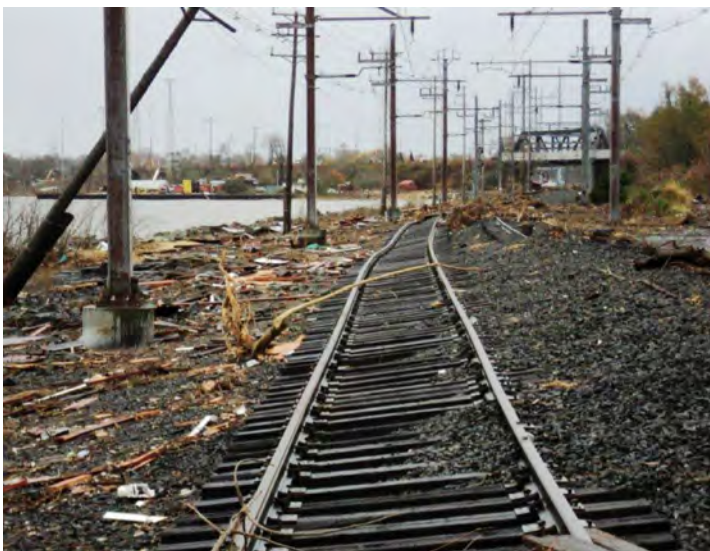
NJT NORTH JERSEY COAST LINE BETWEEN SOUTH AMBOY AND MATAWAN STATIONS.
