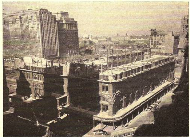
Six months later: Demolition is slow because old station was strongly-built. In background at left is Suburban Station Building
