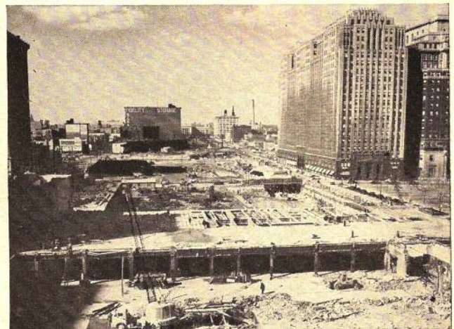
Looking toward 30th St. Station at remains of Chinese Wall. The excavation at right is for additional Suburban Station tracks
