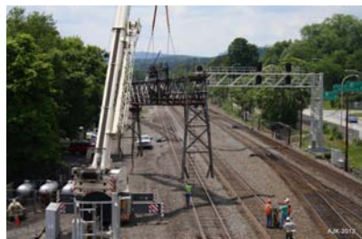
PRR POSITION LIGHT SIGNAL BRIDGE IS REPLACED WITH COLOR LIGHT BRIDGE. JUNE 16, 2012.
