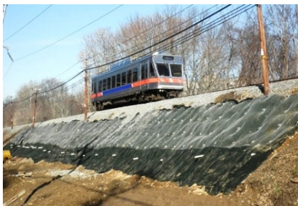
SEPTA EMBANKMENT WORK BETWEEN ROBERTS ROAD AND GARRETT HILL STATIONS. SEPTA PHOTO.
