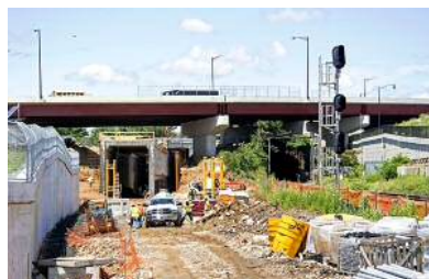
THE OLD VIRGINIA AVENUE TUNNEL, AT RIGHT, WILL BE REPLACED ONCE THE NEW BORE ENTERS SERVICE LATER IN 2016 - BRIAN SCHMIDT
