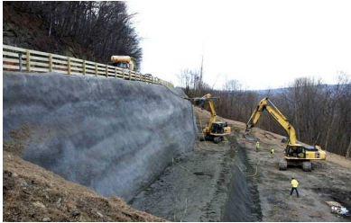
A NEW RETAINING WALL AT WOODCOCK HOLLOW ALONG THE WESTERN MARYLAND SCENIC RAILROAD. THE RAILROAD'S TRACKS ARE ABOVE THE WALL - WESTERN MARYLAND SCENIC RAILROAD
