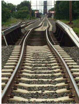
NJ TRANSIT OFFICIALS TOOK THIS PHOTO SHOWING DAMAGE TO ITS BRIDGE AND RIGHT-OF-WAY.
