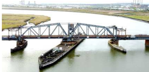
THE PRESENT PORTAL BRIDGE IS SUBJECT TO MECHANICAL FAILURE AND HAS BECOME UNRELIABLE IN RECENT YEARS.
