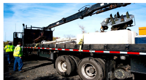
A NORFOLK SOUTHERN CONTRACTOR HAS REMOVED A POSITION LIGHT SIGNAL FROM THE PENNSYLVANIA RAILROAD ERA ALONG THE MAIN LINE BETWEEN HARRISBURG AND ALTOONA, PA. - DAN CUPPER
